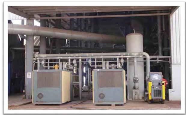
Fig. 1: Grit Recovery System
