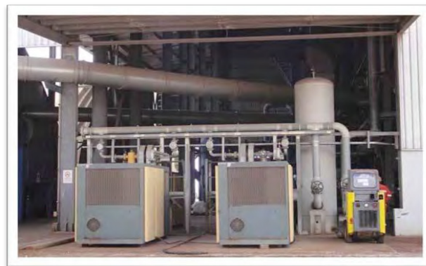
Fig. 1: Grit Recovery System
